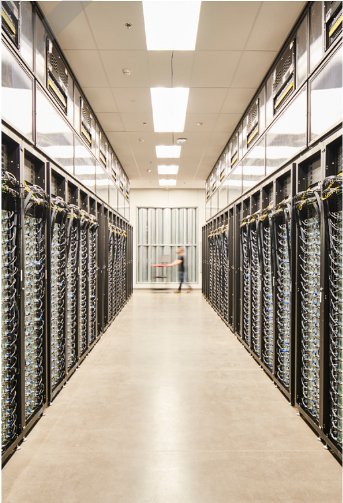
Apple’s Reno data centre, opened in 2012, takes advantage of the mild climate by cooling its servers with outside air whenever possible.
